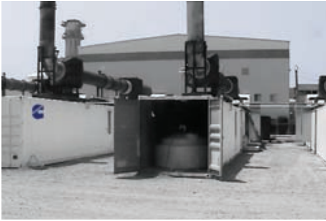
Each unit includes a 600-gallon tank for the urea injection system that controls nitrogen oxides.
