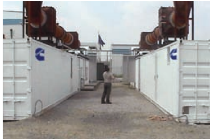
The generator enclosures feature enhanced exhaust silencers and acoustic insulation to reduce noise.
