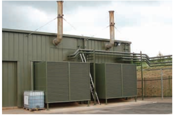
The conduit coming out of the power building contains the 11 kV transmission line that powers the cement plant.
