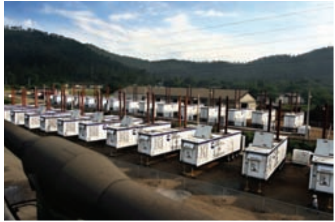
Thirty-two Rental Power units from Cummins Power Generation supplied 64 MW during maintenance on the thermal power plant.
