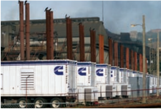
The use of Rental Power from Cummins Power Generation allowed the mine to continue at full production while steam turbines were serviced.
