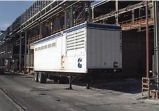
This is one of 11 trailerized emergency Rental Power units installed at Industrial Minera Mexico.
