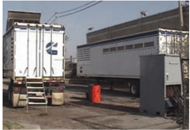
Some generator sets were paralleled to provide power for separate zones within the zinc refinery and the copper refinery.
