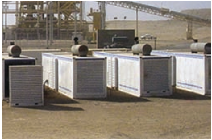
Seven 1000 kW Rental Power units were installed to meet power needs.
