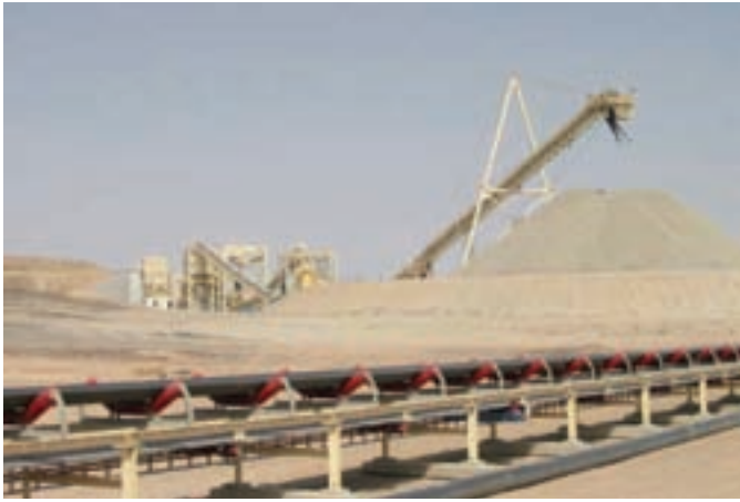
The Rental Power units supply power to run a massive conveyor system and all other electrical equipment used at the mine.
