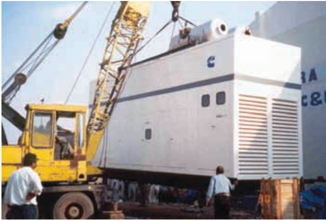
Containerized Rental Power units were customized for acoustics and other customer needs.
