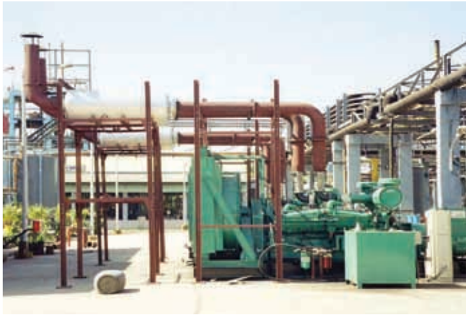
The Rental Power units were fully synchronized with the plant's existing 16 MW turbine power plant to avoid costly downtime.
