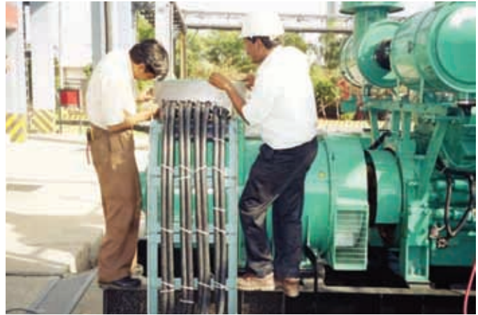
The two 1000 kW units were installed just 25 days after the order was placed.
