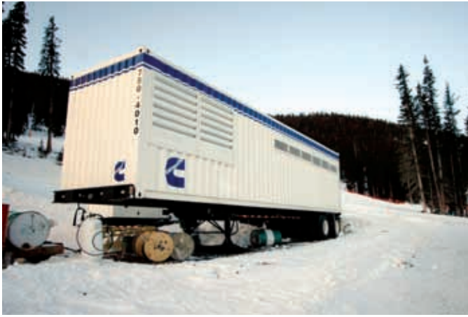
A 750 kW Rental Power unit is used exclusively to supply power for the snowmaking equipment.
