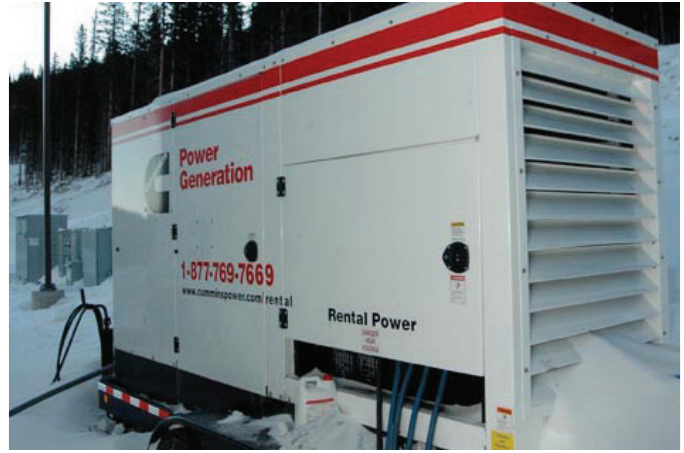
A 230 kW Rental Power unit supplies all the power for the lodge, chairlift and lighting for nighttime snowboarding.
