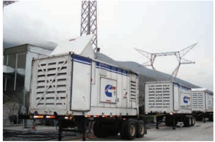
Eleven 1 MW and two 2 MW trailerized Rental Power units provide 15 MW of power to the plant during equipment testing and startup.
