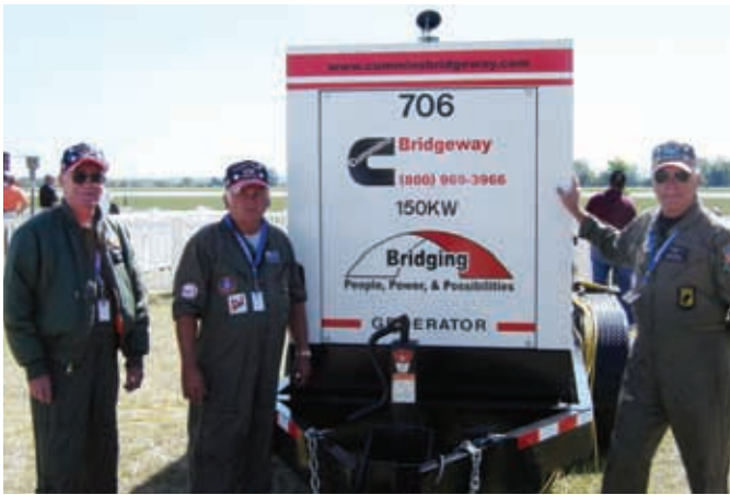
Cummins Power Generation provided 42 Rental Power units for the event through its distributors in Ohio, Michigan and Kentucky.
