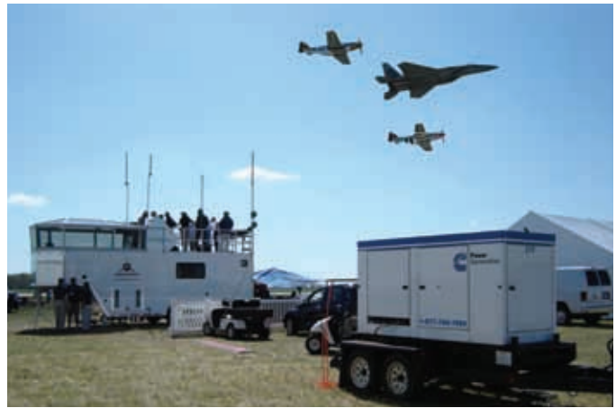
The temporary control tower for the air show was powered by a 250 kW Rental Power unit from Cummins Power Generation.
