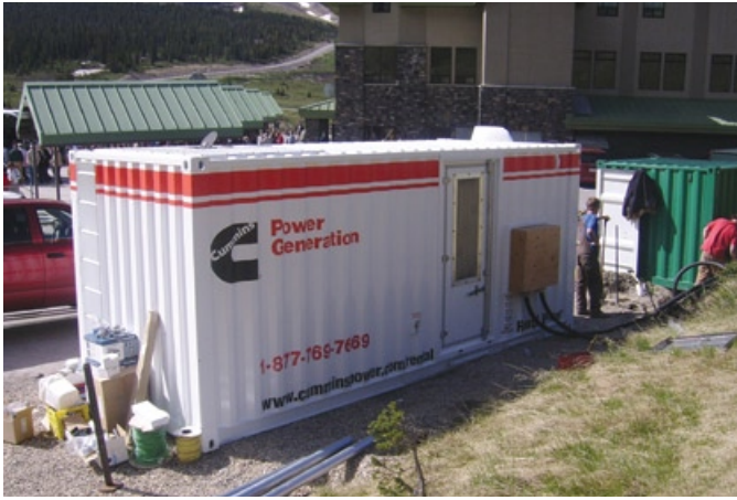
One of the three 500 kW Rental Power units was used for standby power at the Brewster Columbia Icefield Center.
